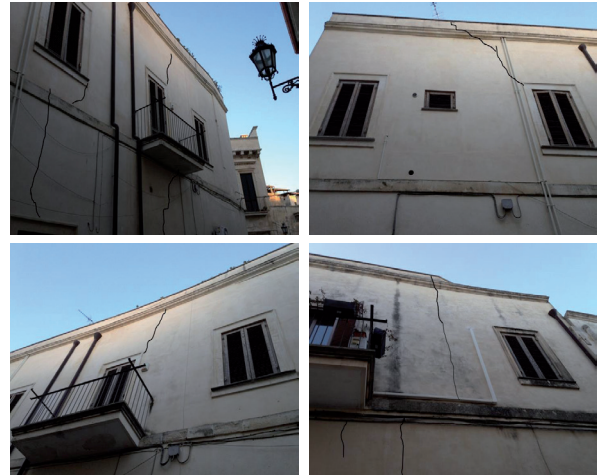
Figure 13. Cracks on the external walls.
